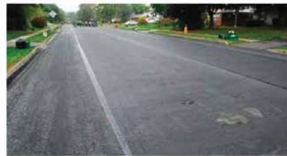
The paving fabric is placed over a leveling course, which is done the previous day to allow the roadway to cool prior to applying the sealant and paving fabric.
