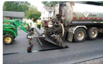
The paving fabric distributor truck sprays PG 64-22 sealant followed by placement of the paving fabric by the spreader/broom tractor unit.
