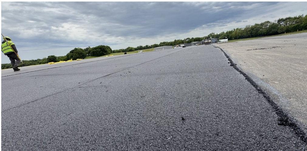
New ARMI + ACE XP overlay placed over the existing runway — Cynthiana-Harrison County Airport, KY
