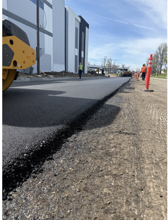
Compaction of the fresh ACE XP-reinforced mat along the new industrial frontage.
