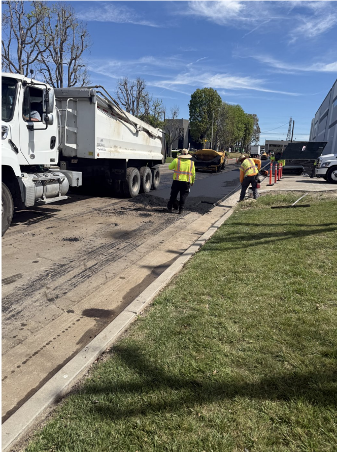
Crew and haul truck staging on the prepared subgrade ahead of paving.
