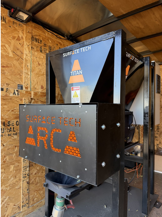
Surface Tech's TITAN dosing system installed at Vulcan Materials' Santa Ana plant.
