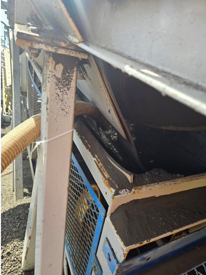
Fiber dosing equipment integrated at Inland Asphalt's plant.
