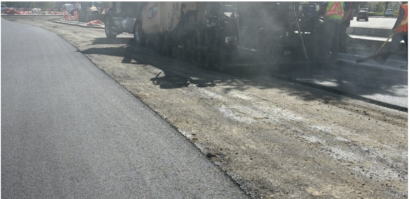
Amrize's paving train placing the ACE XP-reinforced mix on the Beaver Creek Road corridor
