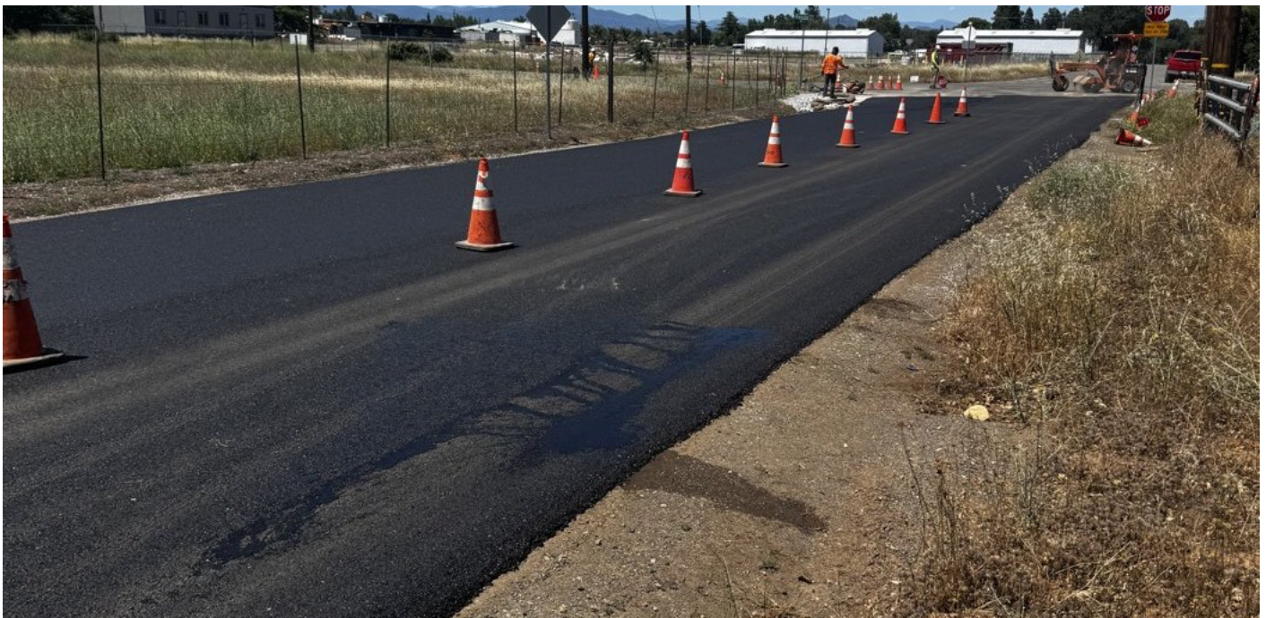
The finished ACE XP-reinforced overlay on Venture Parkway — placed in a single day
